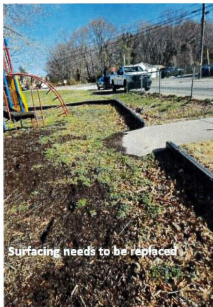
CP 3 Weeds in surfacing
